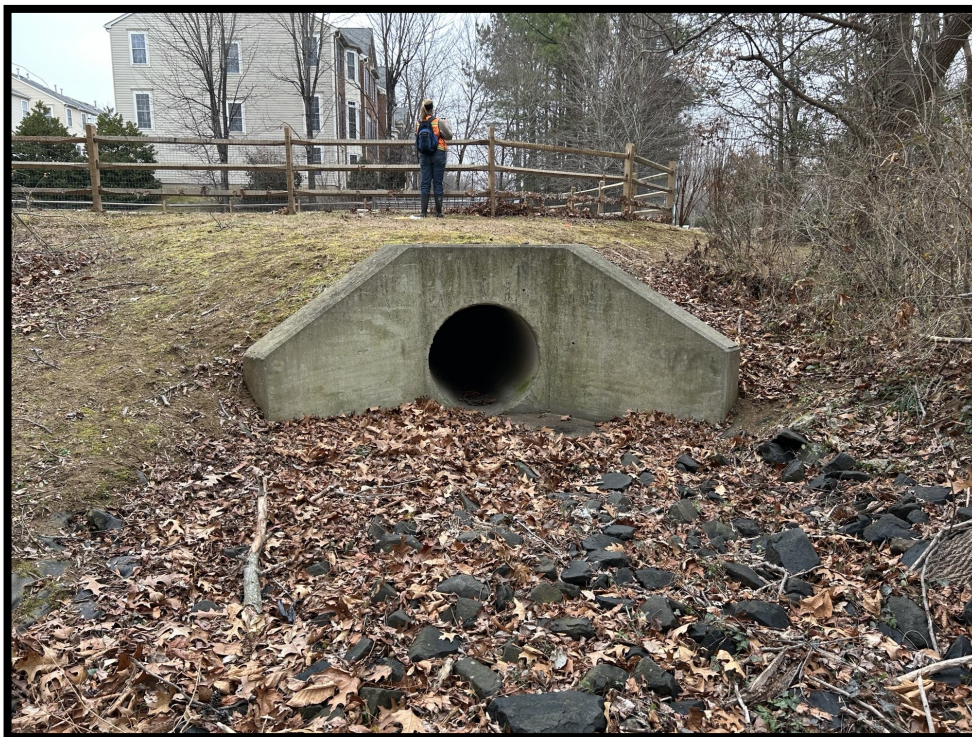
PHOTO 12: SWM pond outfall and rock apron.
