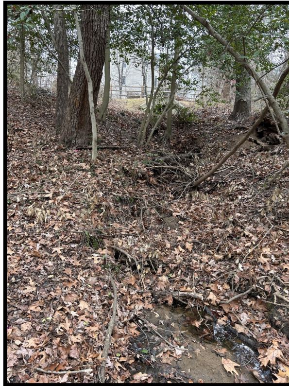
PHOTO 11: Eroded flow path below outfall from SWM pond on left (north) bank.
